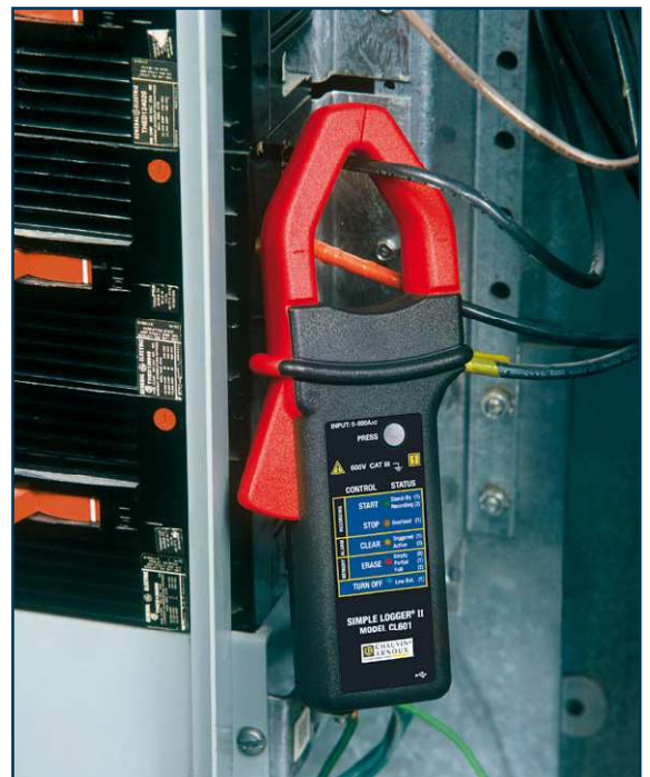
Easily log current in power panels.
